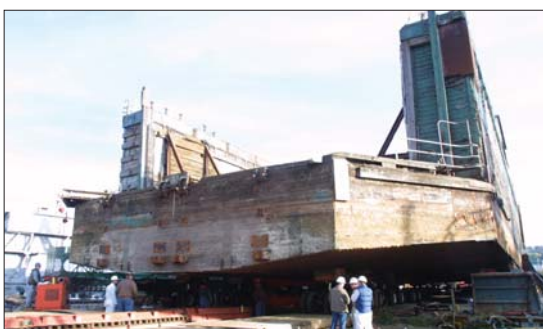
Level wooden runways were built at Foss Terminal to support the old drydock as it rolled slowly from the barge.
