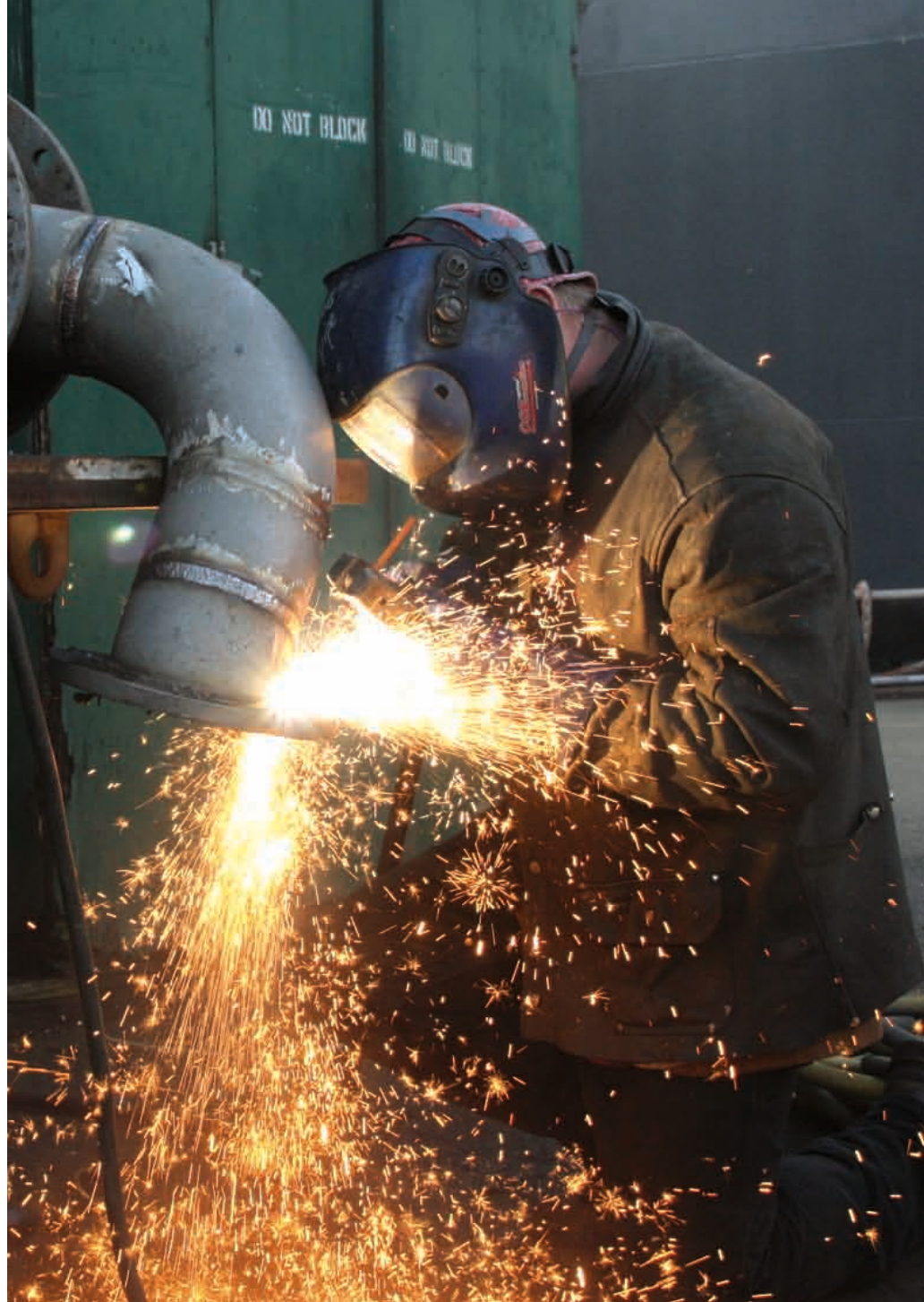
Welder Dane Blanton works on a project at Foss Shipyard in Seattle.
