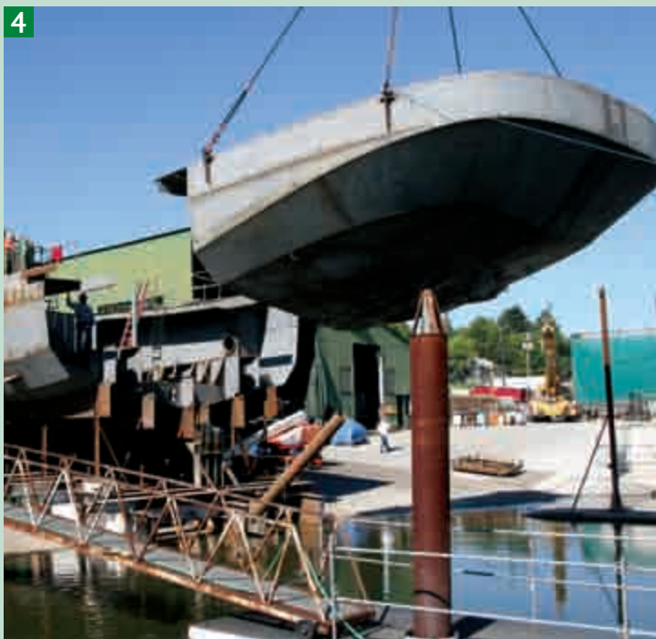
4 The stern section is moved into position on the ways, where it will be welded to the already-placed bow- and mid- sections.
