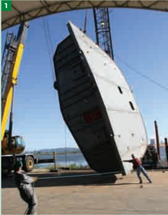
1 The 84,000-pound stern section of the tug, built upside down, is flipped in preparation for transport to the ship ways and union with the rest of the hull.
