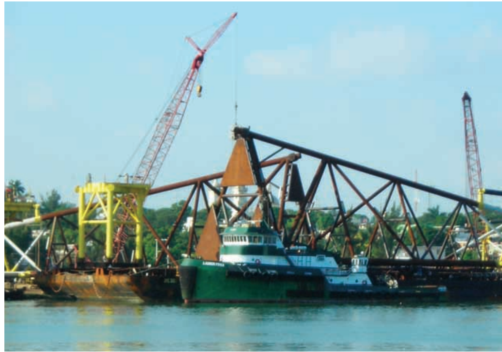
The Lauren Foss and its barge are moored at the Commsa fabrication yard in Tampico, Mexico. On the barge is a 237-metric-ton pipe assembly called a “tripod jacket,” which is a support leg that will rest on the sea floor as part of the offshore platform's structure.
