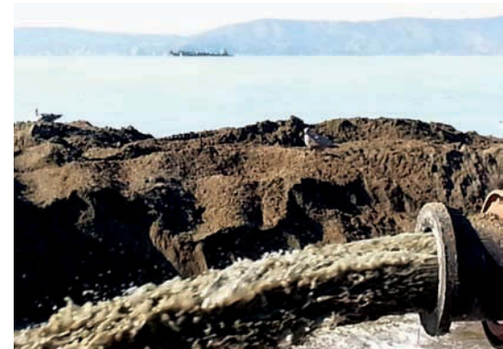
A pipeline carries a slurry of sand dredged by Foss from a barge anchored 7,000 to 10,000 feet offshore. That barge, the Foss dredge and the tug San Joaquin River are visible in the distance.
